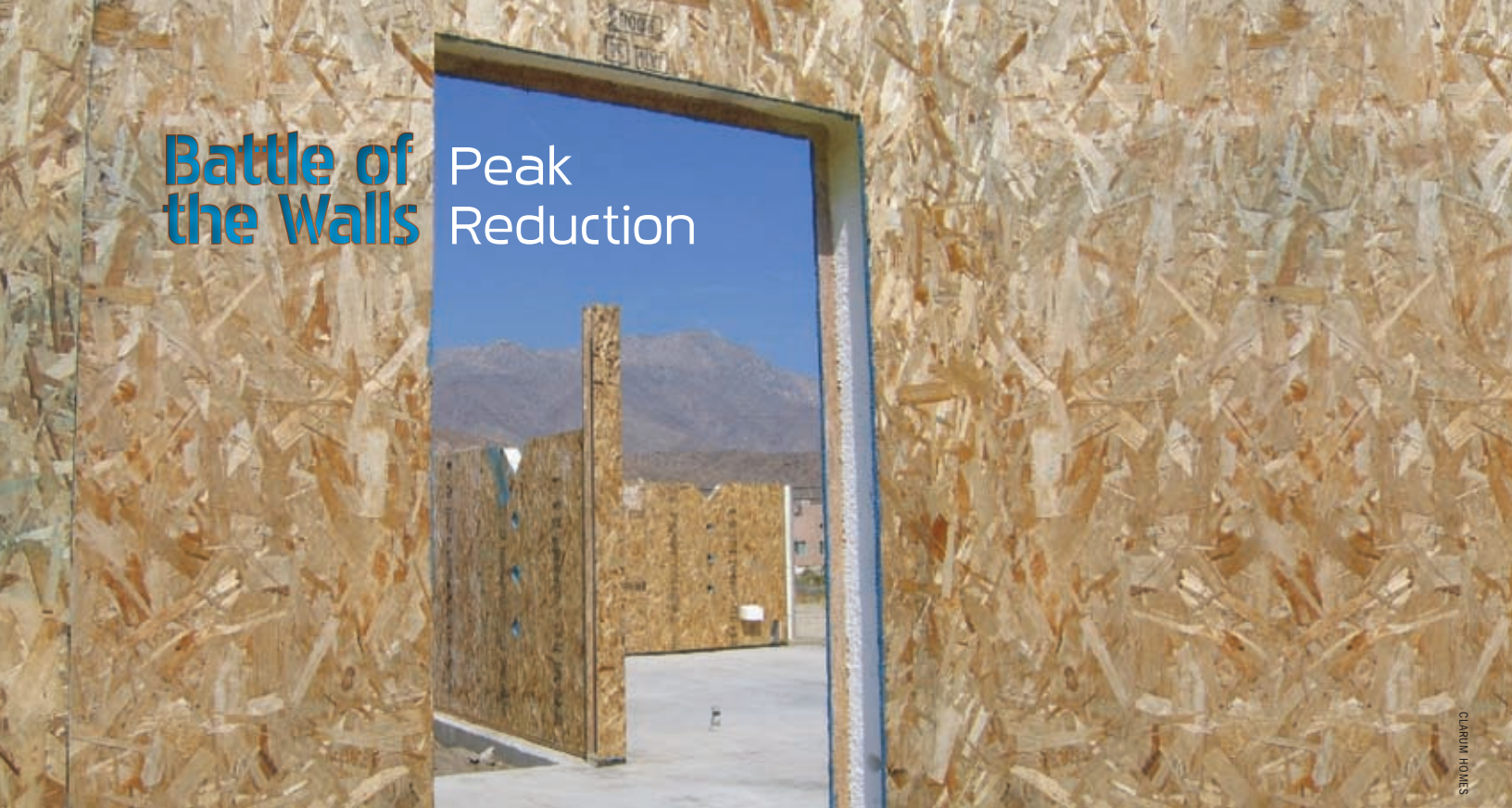
DOE and Clarum Homes teamed up to compare the energy performance of three wall types in three new homes, including the home built with structural insulated panels (SIP) shown in the photo.
